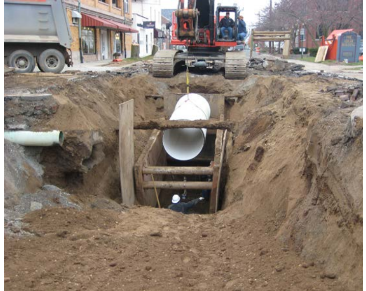
Costly capital improvement projects such as a utility upgrade or road reconstruction should be planned well in advance to ensure adequate funding.
