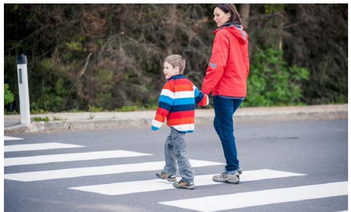
Traditional parallel crosswalk striping can become worn and less visible over time (top). A continental, or ladder, crosswalk is recommended for increased visibility and durability (bottom).
